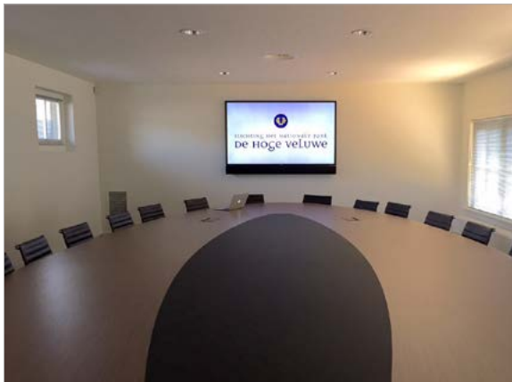
Wall mounted soundbar with 84" screen
